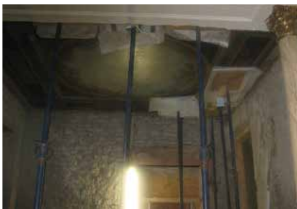
Fig.12 : Painting (b): Security measures taken to avoid the corners of the ceiling to collapse (Photo © Artbee Conservation)
